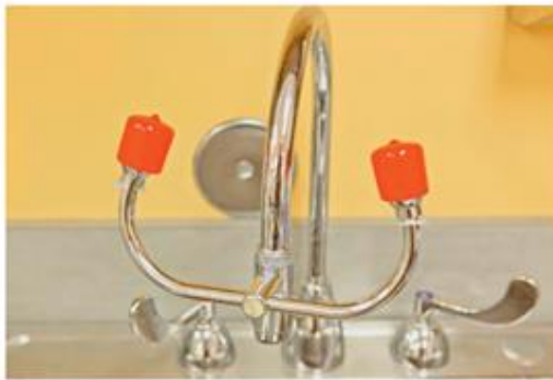
Fig. 1.1 Sink-Mounted Eyewash Station. This type of station is preferable to wall-mounted eyewash bottles that require regular refilling and that may not be of adequate volume to properly flush the eyes.
